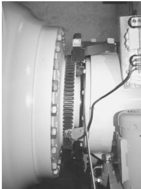
Figure 8.1 Low-speed Shaft Speed Sensing System. (Three proximity sensors mounted on a bracket attached to the front of the (integrated) gearbox register the passage of the teeth on the shaft circumference, and provide independent speed signals for the control and safety systems. The flange onto which the hub is bolted is immediately to the left of the teeth).
